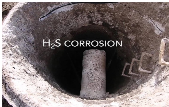
Corrosion caused by hydrogen sulfide
