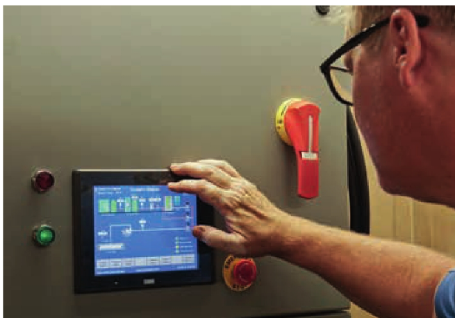
Municipal wastewater technician uses Anue digital monitoring system to control oxygen/ozone injection and view key measures remotely. Photo by Anue
